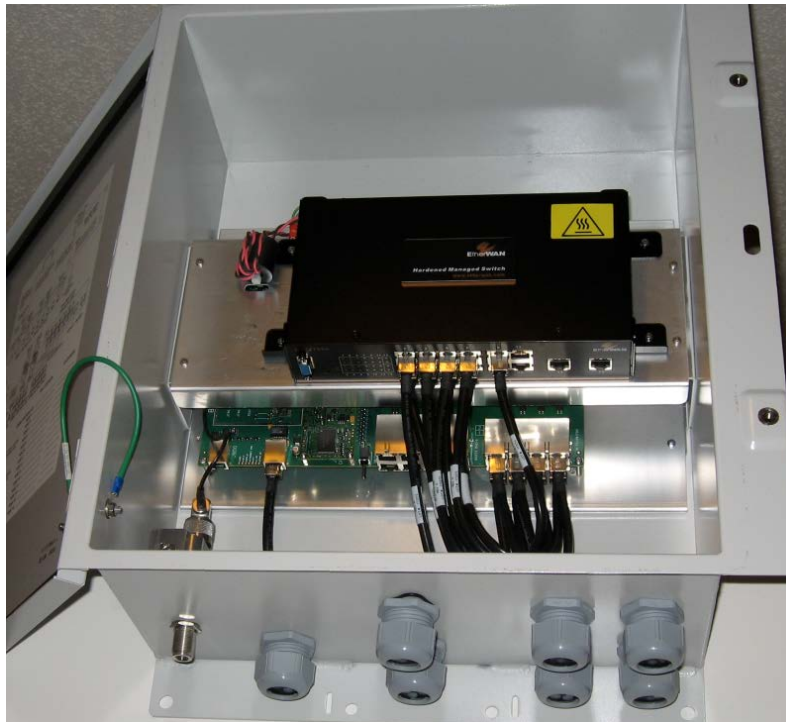
Figure 42 CMM4 (Cabinet with switch)
