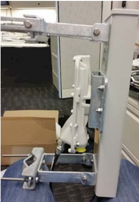
Figure 95 Completed AP and antenna assembly
